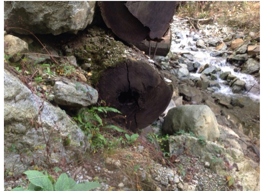
crack in face log on right bank
